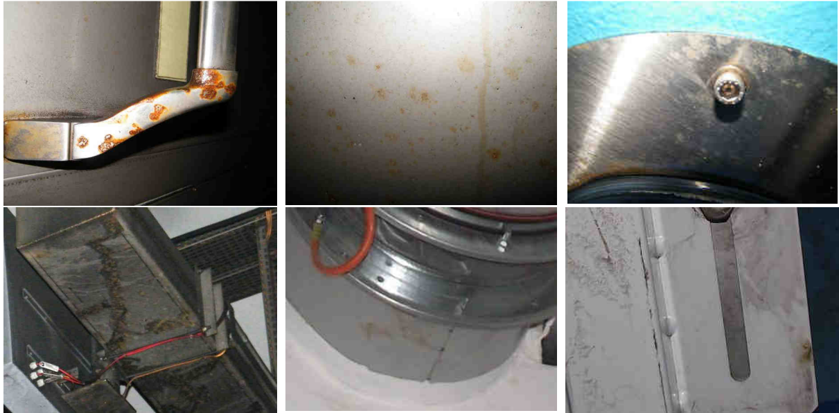
Figure 4: The corrosion attack of materials in tunnel after ½ year service (1 winter season)
