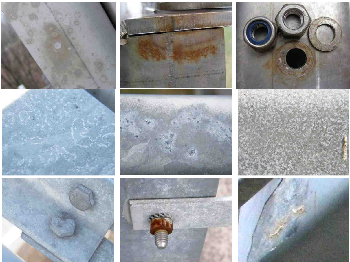
Figure 2: The examples of corrosion on the road infrastructure constructions
