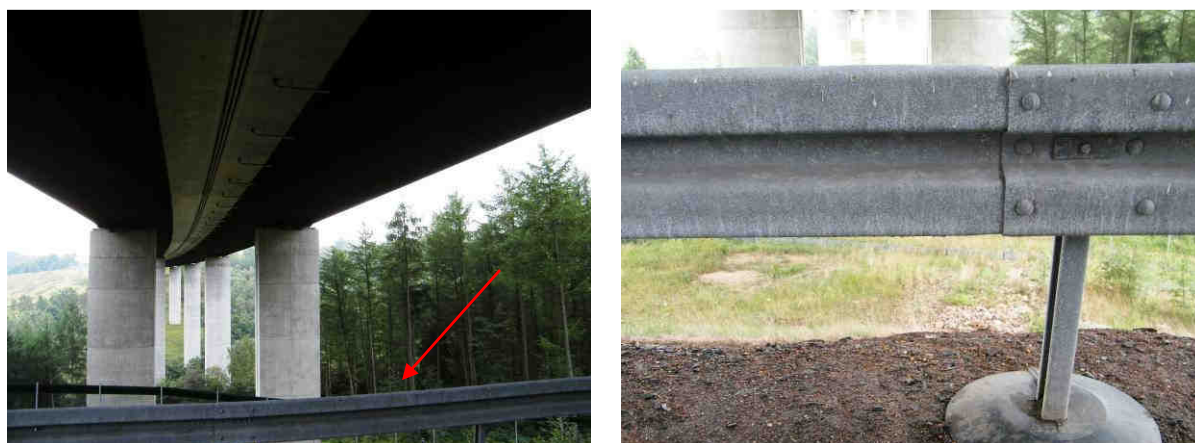
Figure 3: Zinc coating condition on road barriers
